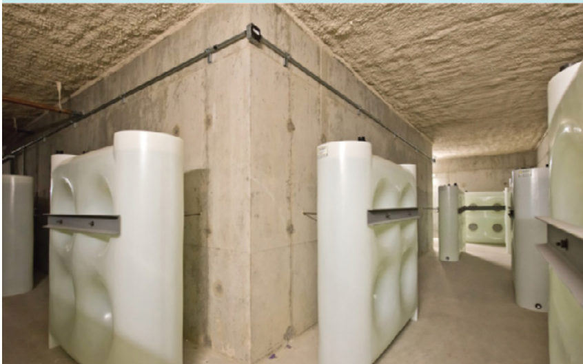
FIGURE 4.9: THE THERMAL LABYRINTH LOCATED IN THE BASEMENT OF THE NEW NANAIMO HOSPITAL EMERGENCY DEPARTMENT BUILDING. WATER-FILLED CONTAINERS INCREASE THE ACCESSIBLE THERMAL MASS.
