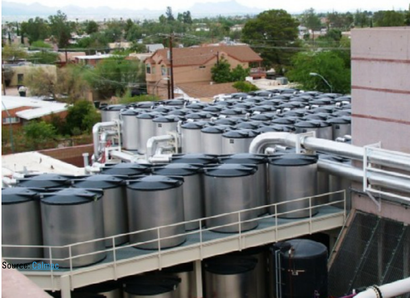
FIGURE 4.6: THERMAL ENERGY STORAGE AT THE UNIVERSITY OF ARIZONA CAMPUS, WITH 23,400 TON-HOURS OF CAPACITY, SERVING 216 BUILDINGS ON A 378 ACRE CAMPUS. INSTALLED IN 2004.
