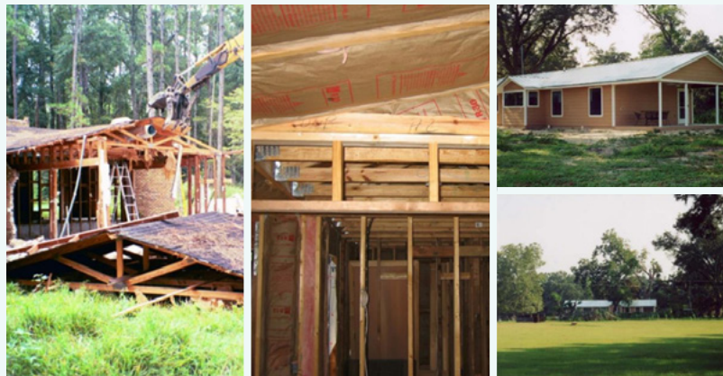
Images of an undamaged 1970s Florida floodplain buyout home being deconstructed. The lumber was used, under existing building codes, to rebuild HUD Section 8 Affordable Housing inland. Photos: Brad Guy
