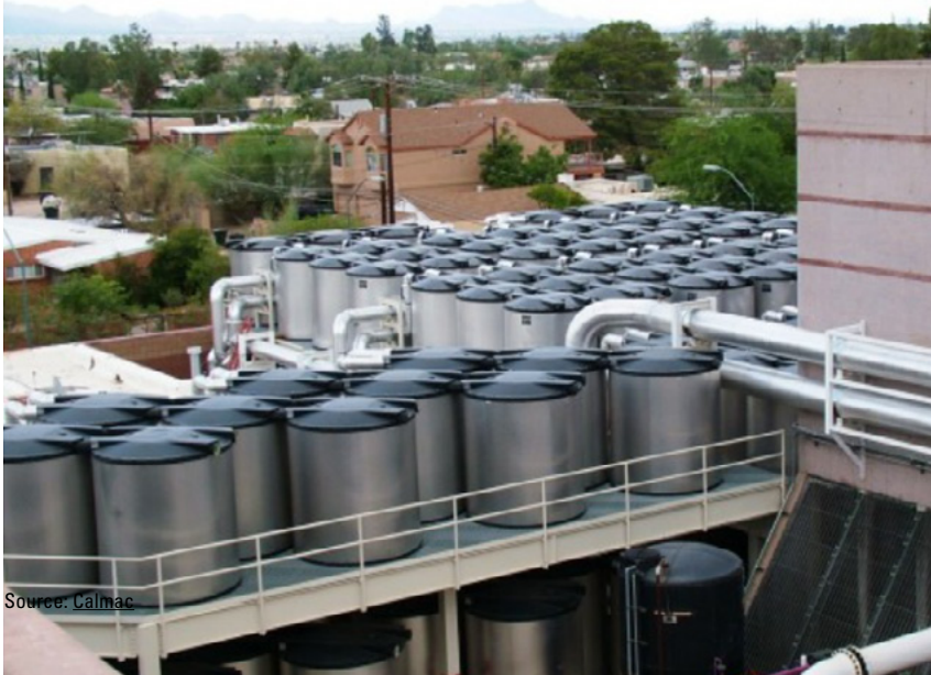
FIGURE 4.6: THERMAL ENERGY STORAGE AT THE UNIVERSITY OF ARIZONA CAMPUS, WITH 23,400 TON-HOURS OF CAPACITY, SERVING 216 BUILDINGS ON A 378 ACRE CAMPUS. INSTALLED IN 2004.
