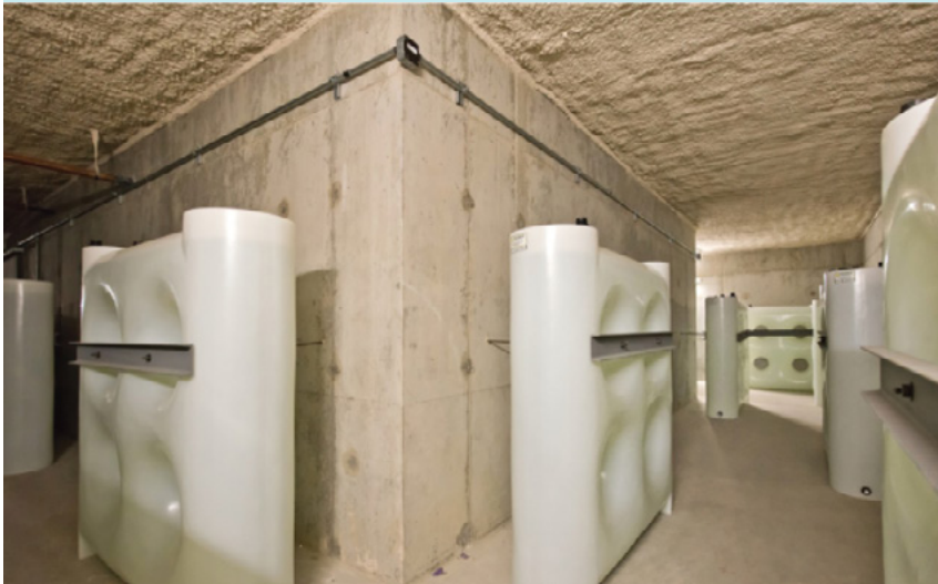
FIGURE 4.9: THE THERMAL LABYRINTH LOCATED IN THE BASEMENT OF THE NEW NANAIMO HOSPITAL EMERGENCY DEPARTMENT BUILDING. WATER-FILLED CONTAINERS INCREASE THE ACCESSIBLE THERMAL MASS.
