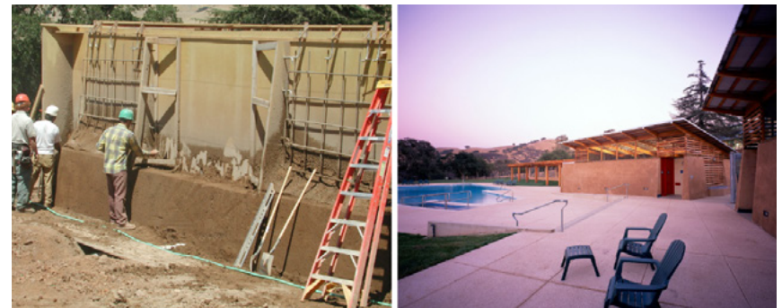
Source: Camp Arroyo, Livermore, CA. Bath House. Stabilized earth construction. Photos courtesy of Siegel & Strain Architects and JD Peterson.
