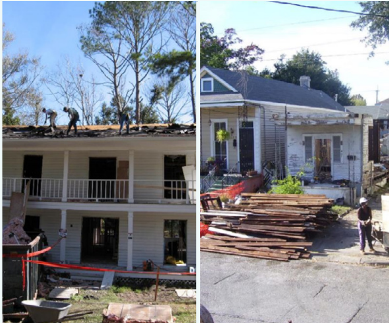
Post-Katrina Mercy Corps deconstruction projects involved a range of materials and home types, from historic to contemporary. Photos: Brad Guy
