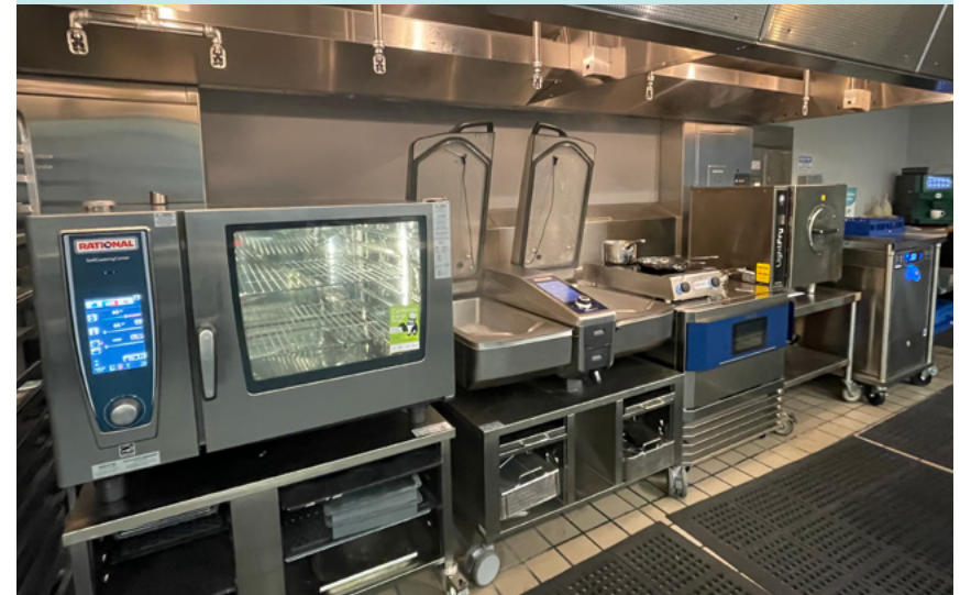
FIGURE 5.19: A HIGH TECH ALL-ELECTRIC KITCHEN LINEUP WITH COMBI OVEN, INDUCTION COOKTOP, FLEXIBLE BRAISING PAN, BLAST CHILLER, HOT AIR FRYER, AND HEAT RECOVERY DISHMACHINE
